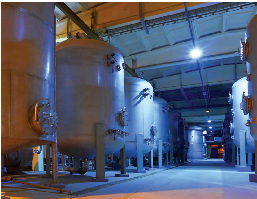
Image 8. Hydrogen gas storage is integral to the gas supply industry
